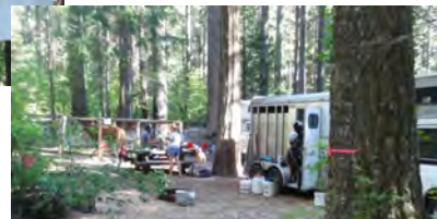
Equestrian volunteers from Gold Country Trails Council constructed these permanent horse pens at Skillman Horse Camp. Many thanks to GCTC.
