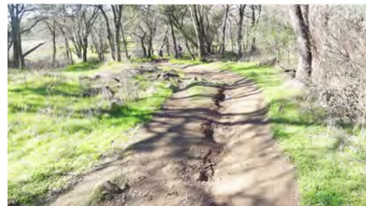
Severely rutted Center Trail with incised fall-line with (improper) drainage. The new Center Trail is parallel to the original trail, and will have proper out-slope drainage.
