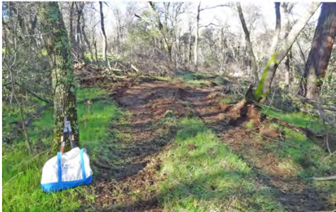
First-Pass by Heavy Equipment. Cut Branches to be Repurposed for Abandonment of the Old Alignment of the Center Trail
